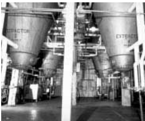
These giant 2,500-gal Cone Screw Mixers have revolutionized oleoresin extraction at Givaudan-Roure's high tech flavor production facility. Equipped for vacuum and heat transfer, they have boosted product yields and consistency, and shortened the process cycle.
